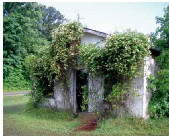
An abandoned store on the Lake Loop.
